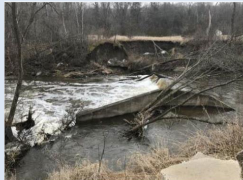
Figure 5: Right Bank Scour
